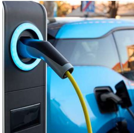
EV CHARGERS AND EXTENSIVE PARKING
